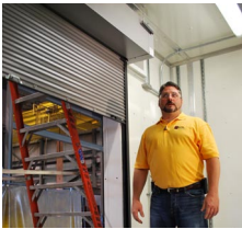
Fusible link drops down fire-rated shutter.
